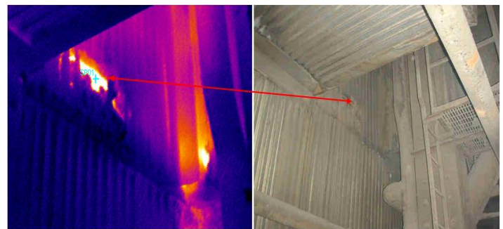
Boiler Tubes defects identification
